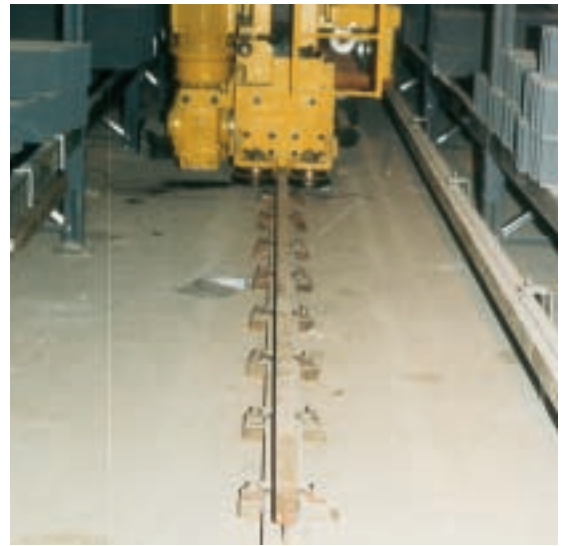
AS/RS Stacker Cranes
