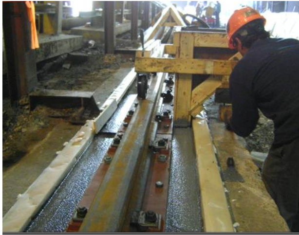
Photo of a typical Head Box used to increase flow across the grout area
