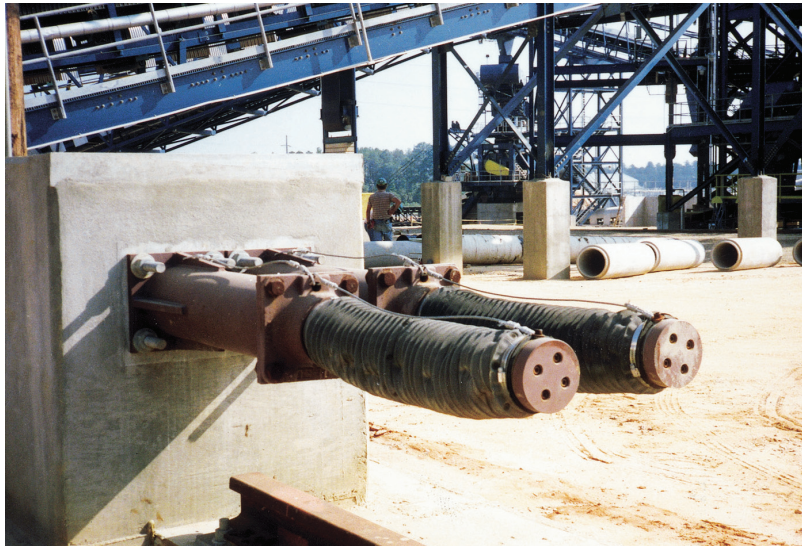
2 Type 76 Bumpers on Stacker/Reclaimer EndStop in Coal Yard.
